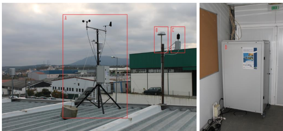
Fig. 1. Set of the monitoring equipment used in the study: (A) Weather station; (B) air intake; (C) smart noise sensor; (D) gas analyzers container.
