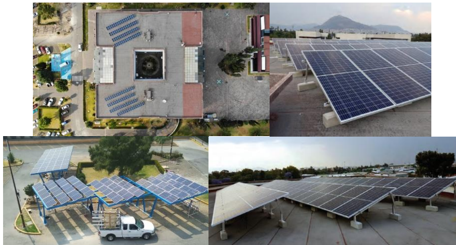
Fig. 7. Solar FV system installed at CIC-IPN.
