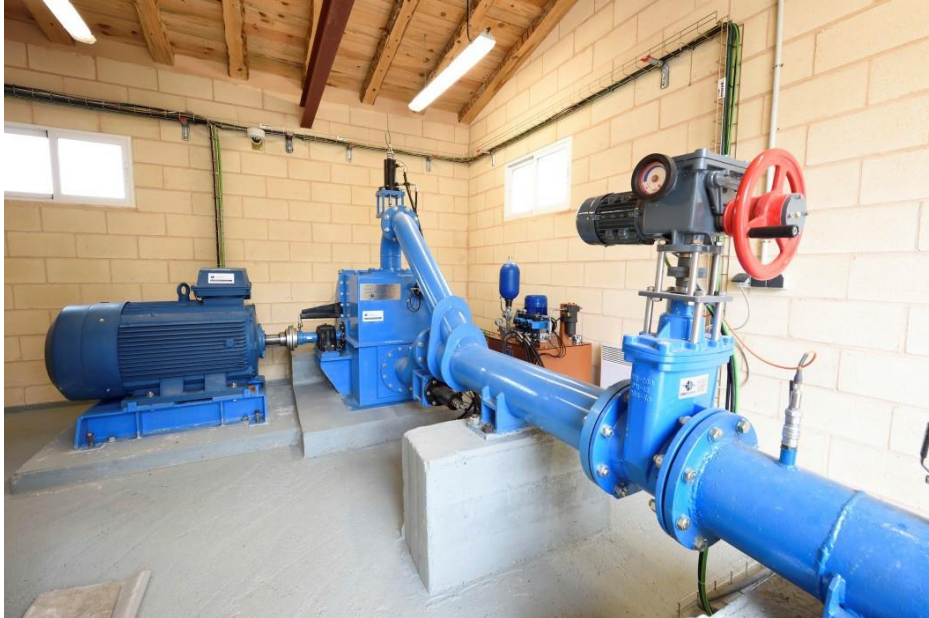
Fig.2. Pelton hydraulic microcentral installation. Courtesy CEDER.
