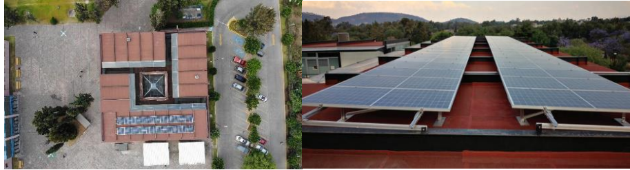
Fig. 8. Solar FV system installed at CIDETEC-IPN.
