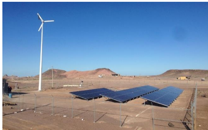
Fig. 1. Microgrid of the community of Puertecitos, Mexico.
