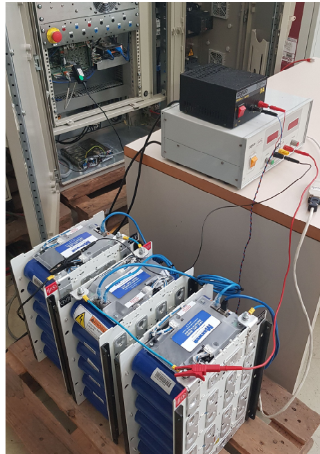
Fig. 4. The three supercapacitor modules connected in series. The maximum voltage is 192 V and the capacitance per each module is 141 F.
