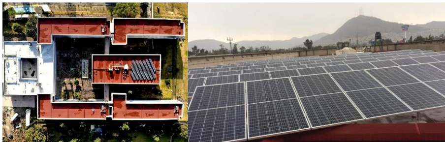
Fig. 9. Solar FV system installed at ESCOM-IPN.
