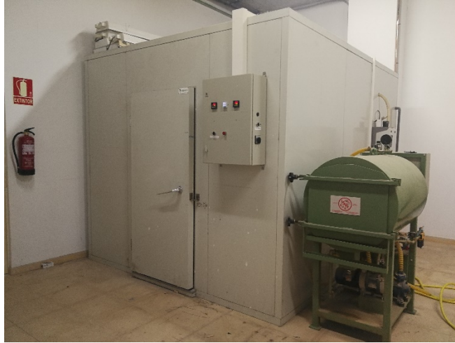
Fig. 1. Temperature and humidity controlled chamber at the EIFAB in Soria, Spain
