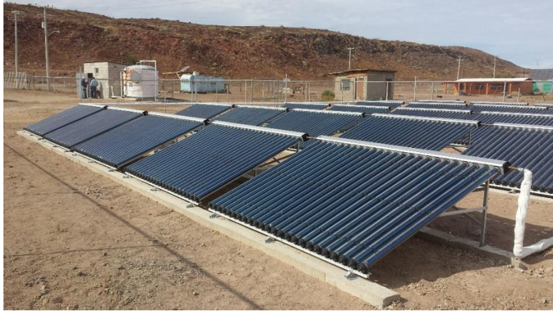
Fig. 2. Thermosolar absorption cooling system of 35 kW capacity installed in the primary school of Puertecitos, Mexico.
