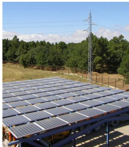
Fig. 2. Photovoltaic system integrated in the rooftop of the parking area of CEDER in Lubia (Soria, Spain). Image courtesy of: CEDER.
