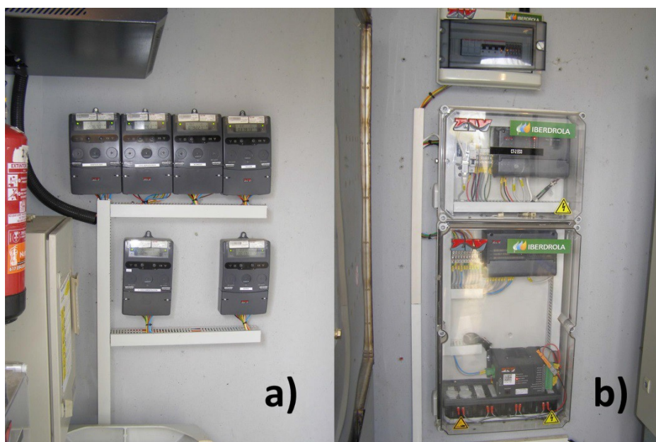
Fig. 5. a) Smart meters for the measurement of consumption and DG ; b) Data concentrator in transformation center to monitor smart meters in low voltage.
