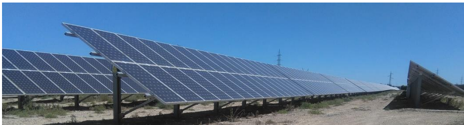
Fig. 3. General image of the 3 MW PV plant in which has been developed the research.
