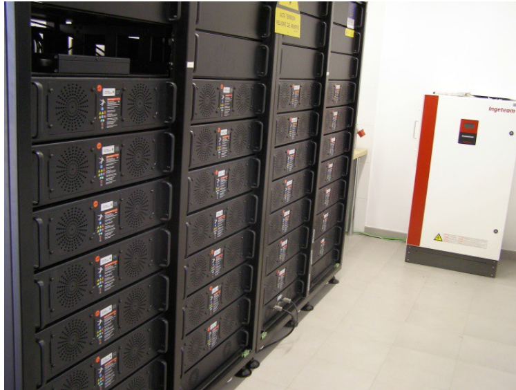
Fig. 4. Lithium-ion battery and bi-directional inverter. Courtesy CEDER.
