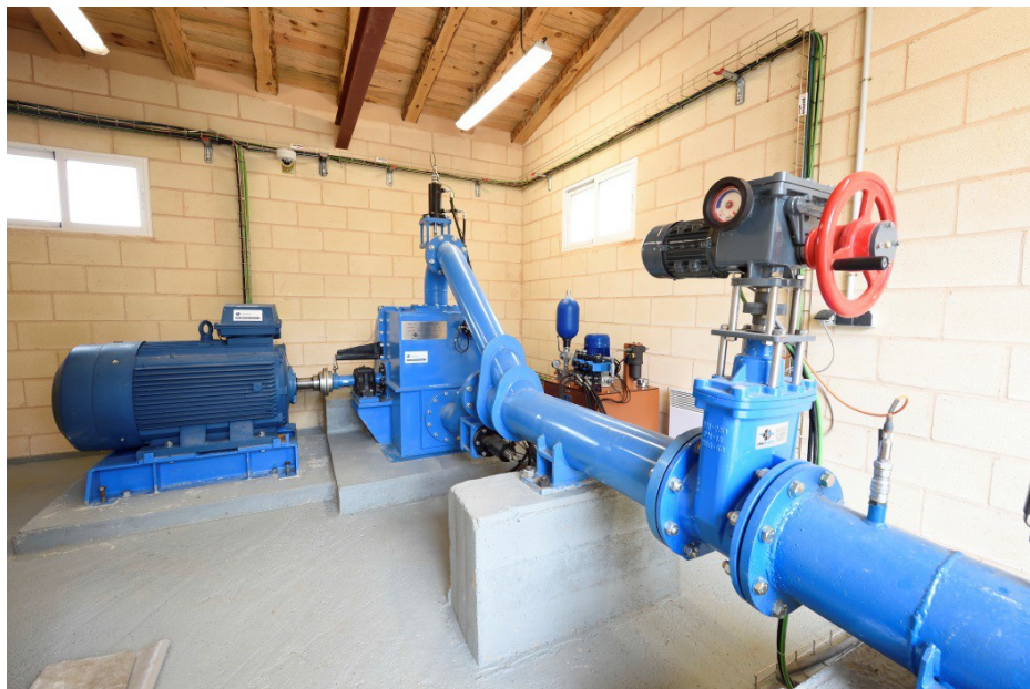
Fig. 3. Pelton hydraulic microcentral installation. Courtesy CEDER.
